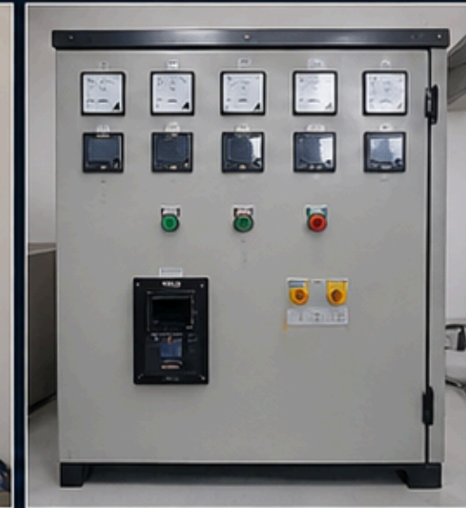
DG SYNCHRONIZATION PANEL
