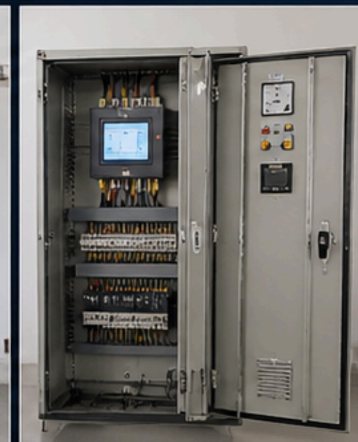
SCADA / HMI PANEL
